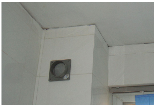
Fig. 6. Cracks between wall and ceiling in Hui'an building in Tangshan.
